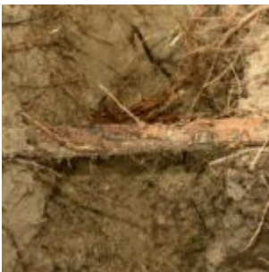
Horizontal root ingrowth in the pipe trench
