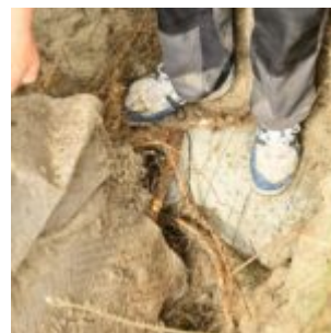
Protective mat, roots and sewage pipe
