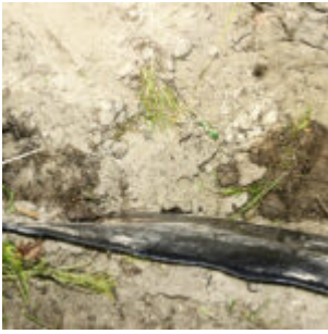
Looking vertically down into the pipe trench: The black protective mat against roots is clearly visible
