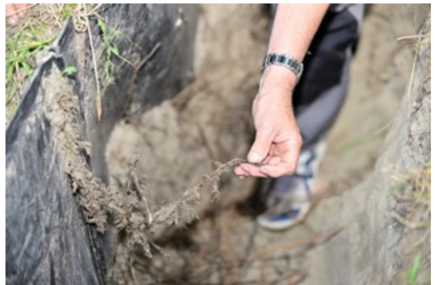
Despite protective mats: Roots continued to grow merrily
