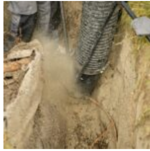
Suction excavator carefully removes soil around sewer pipes without damaging tree roots
