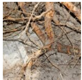
Almost like an ancient Roman trident: tree roots grow towards the sewage pipe
