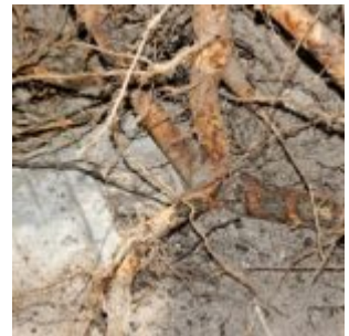
Almost like an ancient Roman trident: tree roots grow towards the sewage pipe
