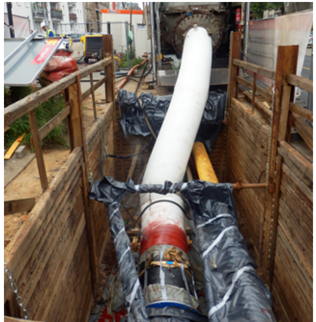
IKT Compare: testing lining systems for the trenchless rehabilitation of pressure sewers
