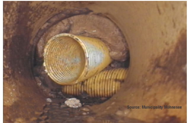
Illegal drainage system connection to a public sewer
