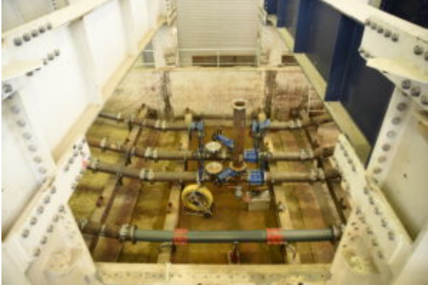
View of the built-in sewer pressure pipelines in the IKT large 1:1 scale test facility
