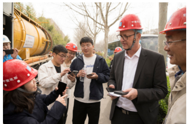
Prof. Dr. Bert Bosseler visits a CIPP liner construction site in Jinan, China
